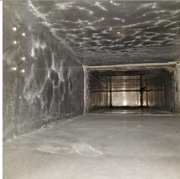
Before 2 nd Horizontal Duct UV Area
