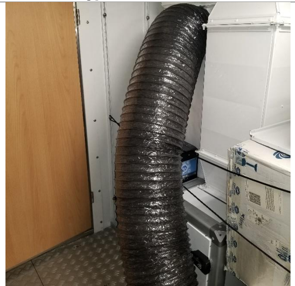
Flex Connected to Main Duct
