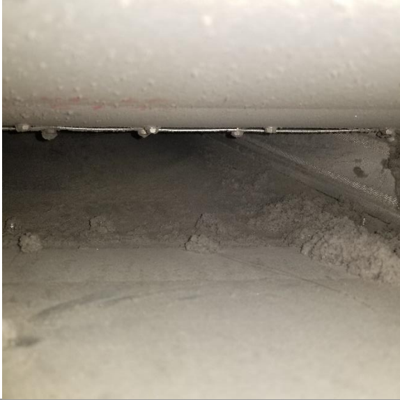
BEFORE Laundry Horizontal Duct
