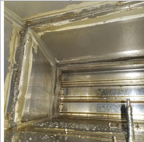
Before Fire Dampers
