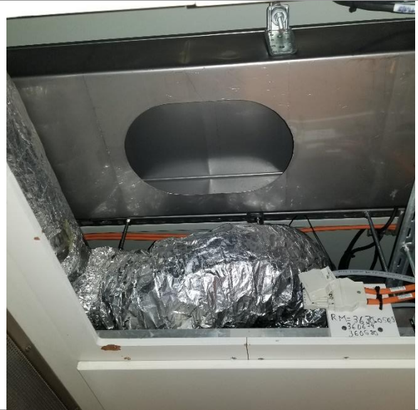
After Exhaust System Access Opened
