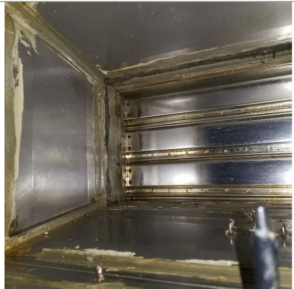
After Dampers Cleaned
