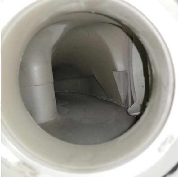
Before Dryer Connection Area
