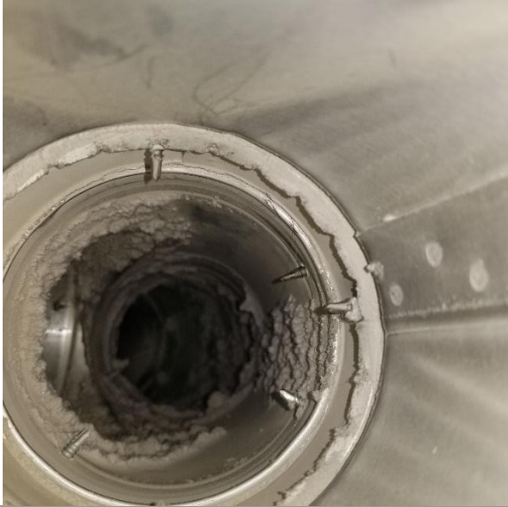
BEFORE Typical Round Duct Dirty
