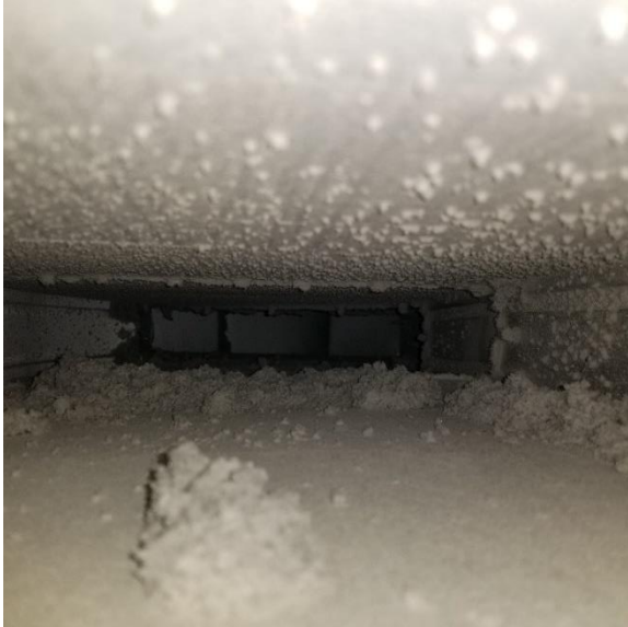
BEFORE Laundry Duct
