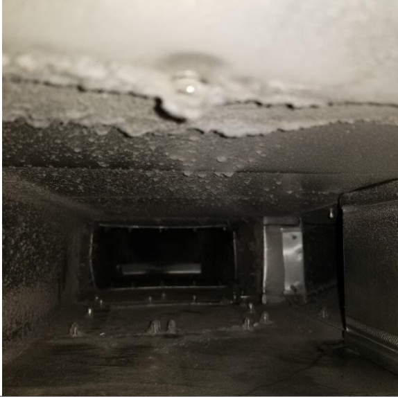
BEFORE Laundry Horizontal Duct
