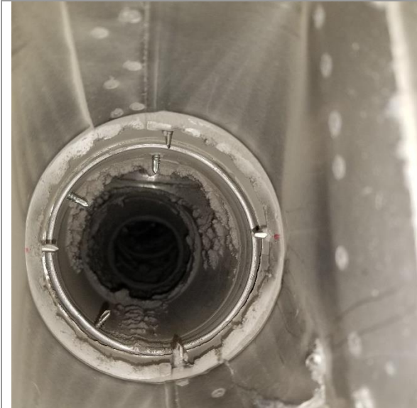
BEFORE Typical Round Duct Dirty
