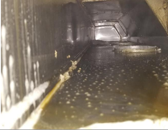
Before Horizontal Duct UV Light Area
