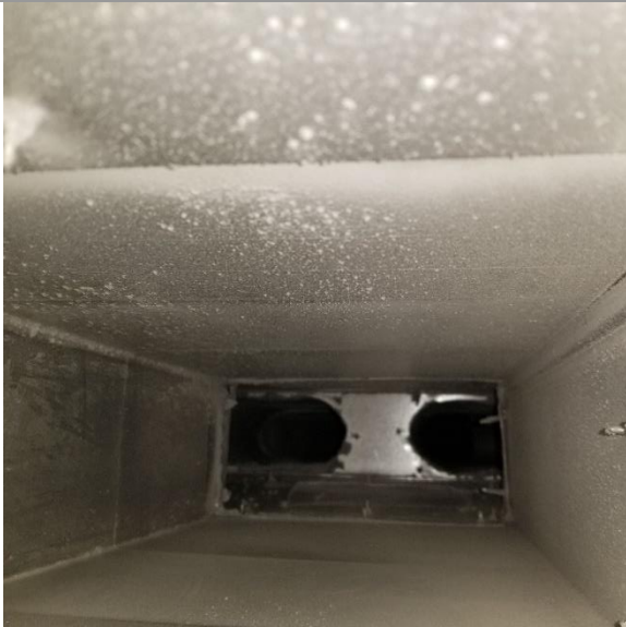
BEFORE Laundry Horizontal Duct
