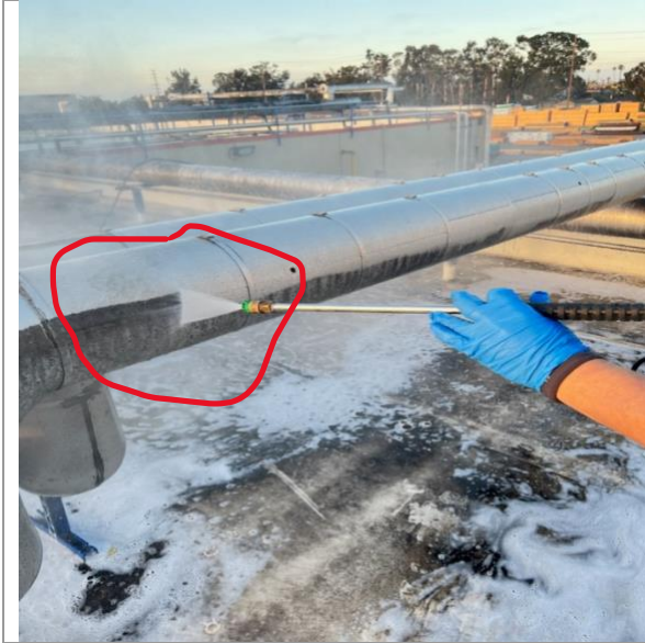
In Cleaning Process All pipes cleaned the same manner with same results (Note Color Difference)
