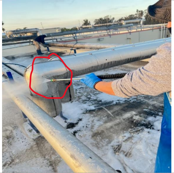
In Cleaning Process All pipes cleaned the same manner with same results (Note Color Difference)
