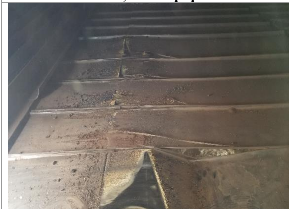
Debris and Some Damage to Metal Interior
