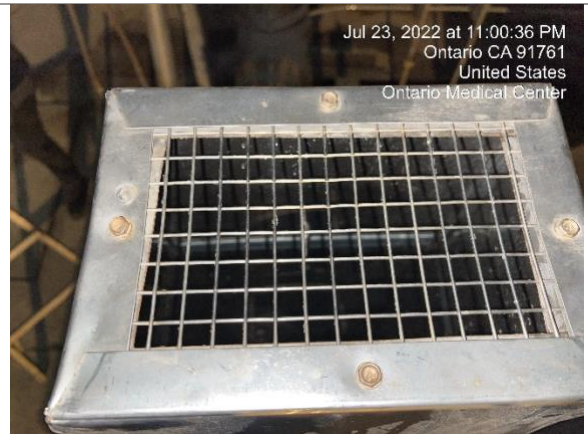
After Exhaust Port on Rooftop
