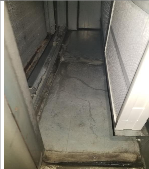
Before Filter Area
