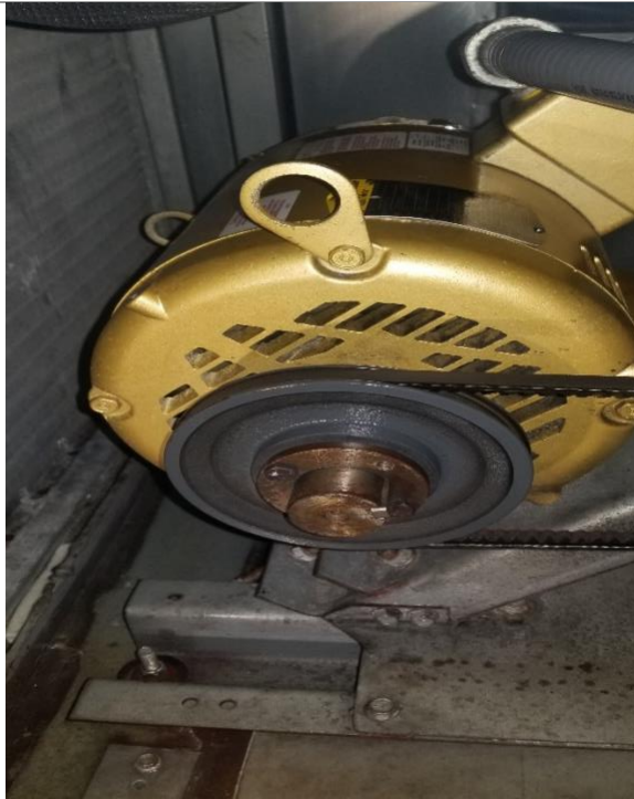
Before Reverse Motor Area – Belt in good condition (Some corrosion observed)
