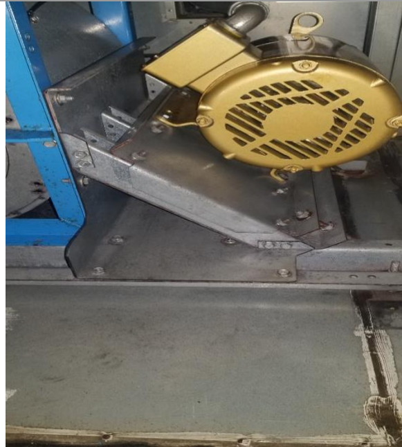
After Interior Fan Motor
