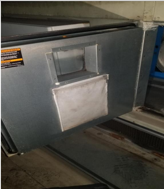
Before Interior of access doors
