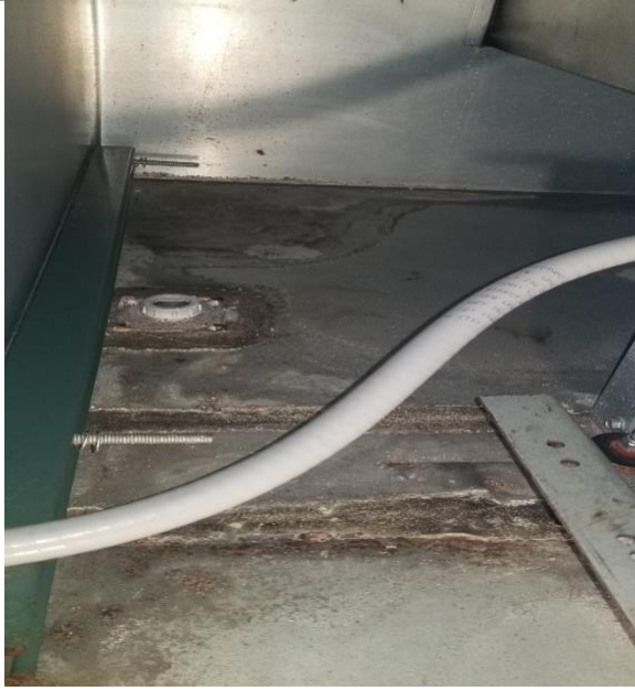
Before Interior of unit with corrosion (Supply Side)
