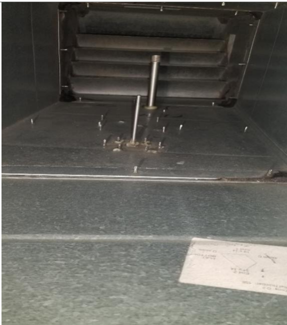
Before Interior Duct with Louvers/Dampers
