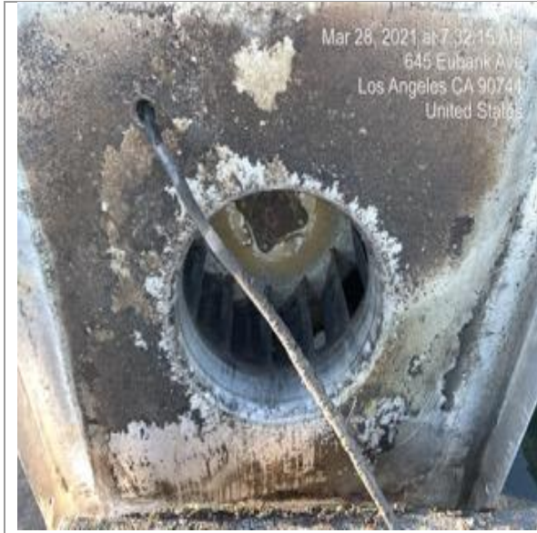
Before Typical Findings for Inner of Fans
