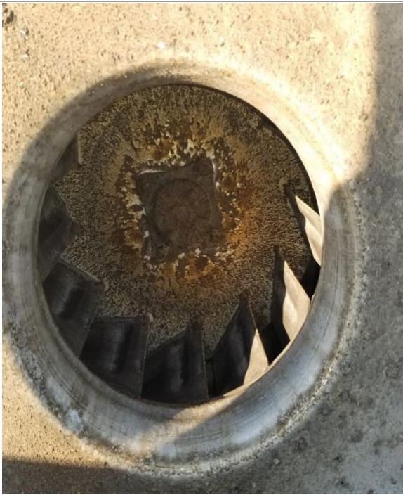
Before Typical Findings for Inner of Fans
