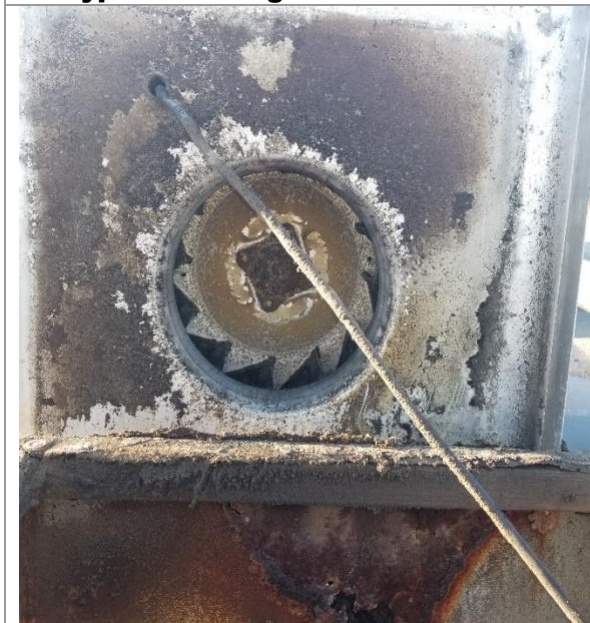
Before Typical Findings for Inner of Fans
