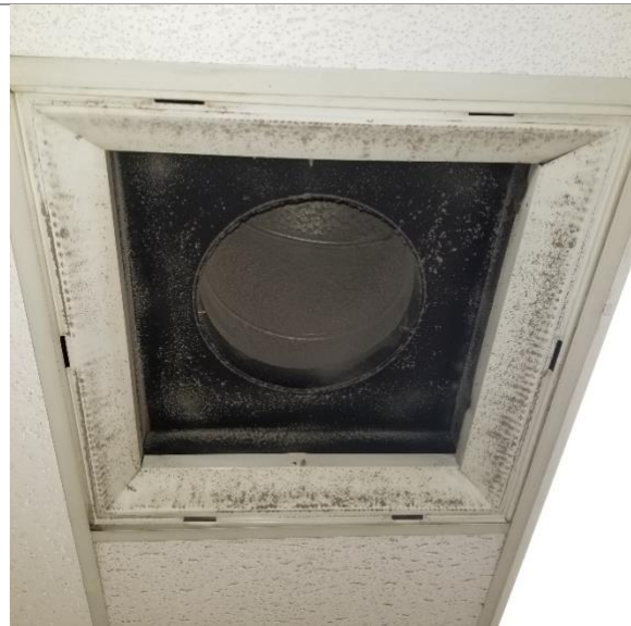
--Before-- Debris on register housing
