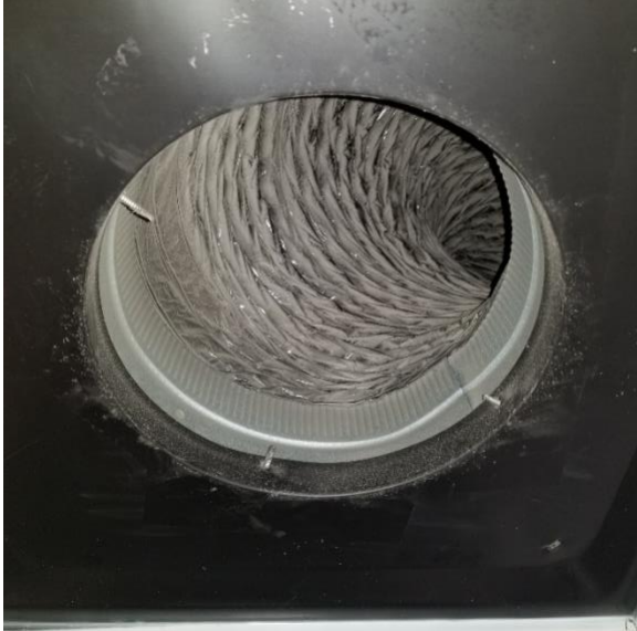
-Before- Dirty flex duct
