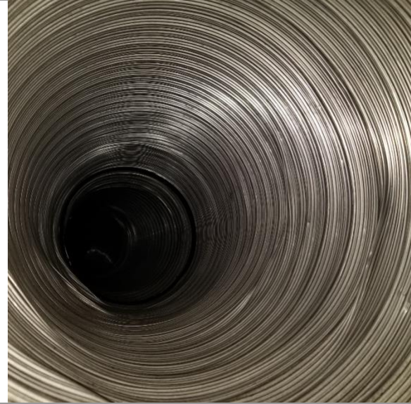
--Before-- Main Duct
