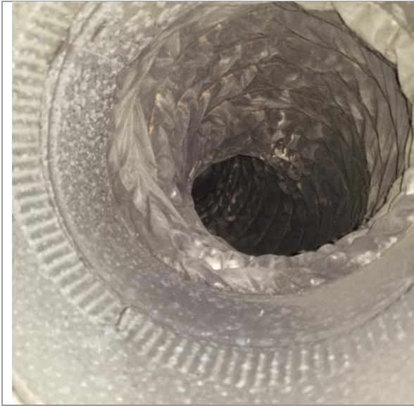
Flex duct deterioration, interior fabric a host for debris
