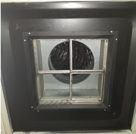
--Before-- Dirty flex duct
