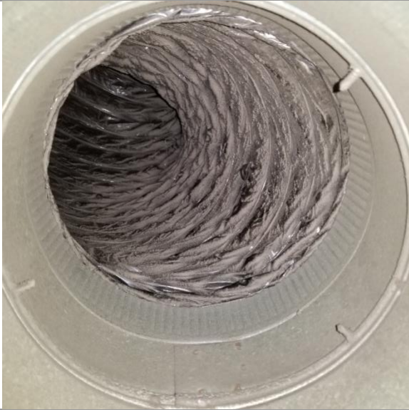
--Before-- Dirty flex duct
