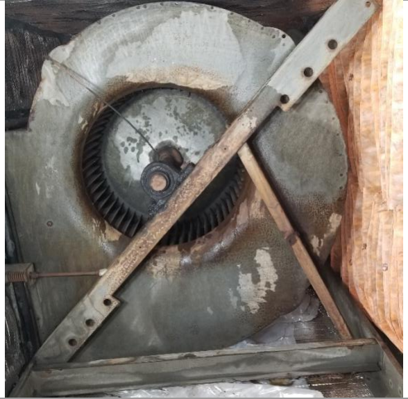
---After--- Unit cleaned
