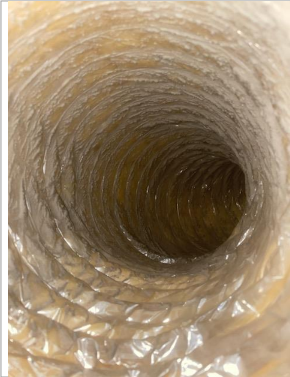
-Before- Dirty flex duct
