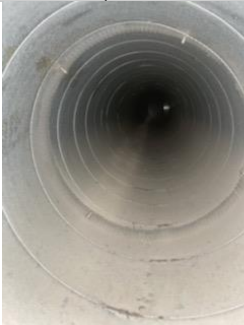
-Before- Dirty main duct
