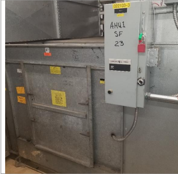
1 st Floor AHU #1
