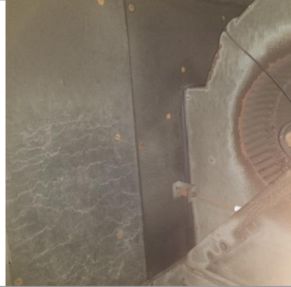
--Before-- Deteriorating insulation is part of cause for debris
