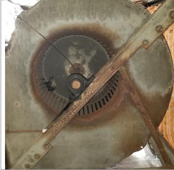
--Before-- Unit with heavy debris and organic growth
