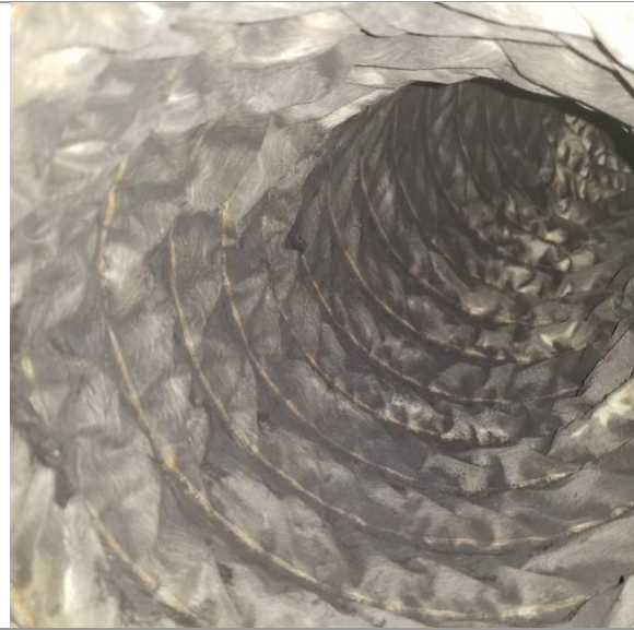
--After-- Difficult to remove debris from these interior fabric flex ducts. Should consider they be replaced. Mostly found in 1 st floor offices
