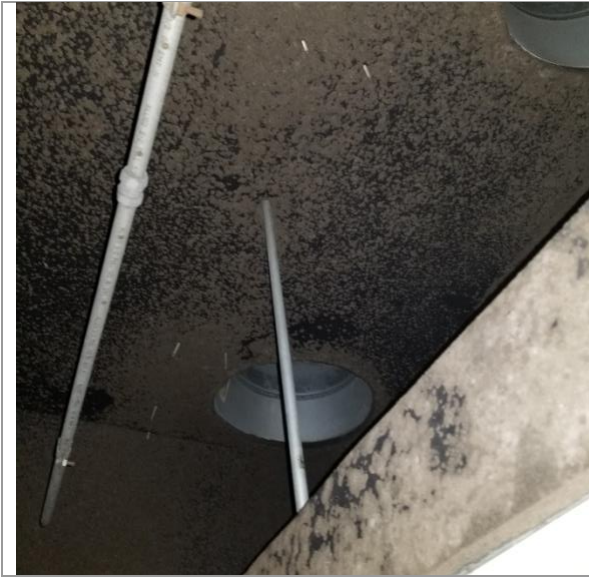
--Before-- Plenum area with debris and organic growth
