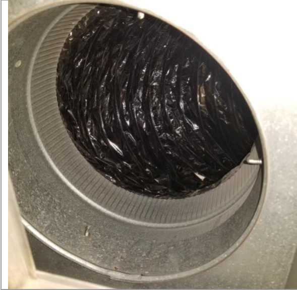
--Before-- Dirty flex duct
