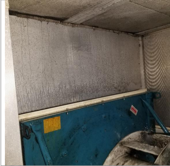
--Before-- Fan area with debris and organic growth
