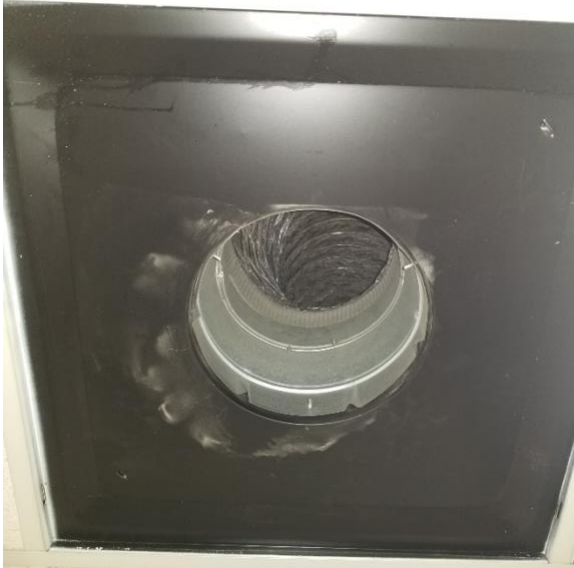
--Before-- Dirty flex duct
