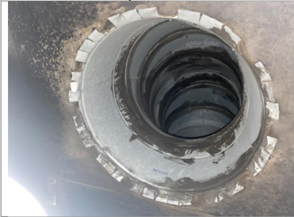
--Before-- Dirty main duct
