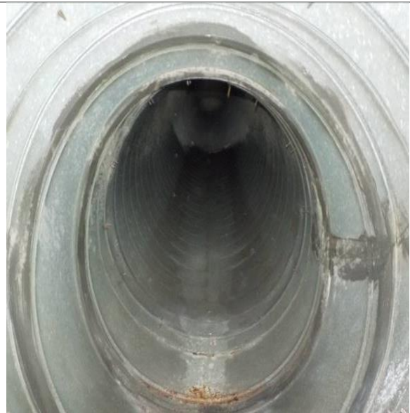
---After--- Sample of Mechanical Area Ducts
