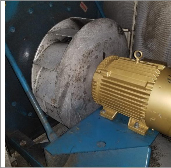
--Before-- Fan with debris and organic growth
