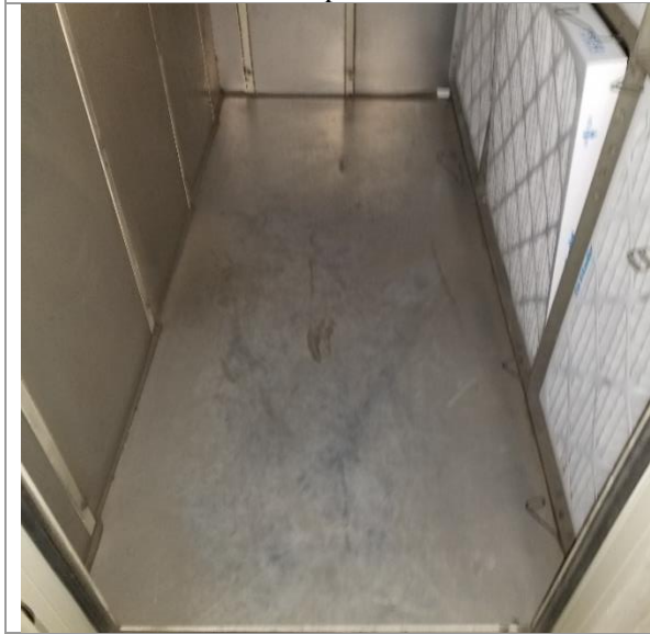
--Before-- Interior of fan compartment with debris
