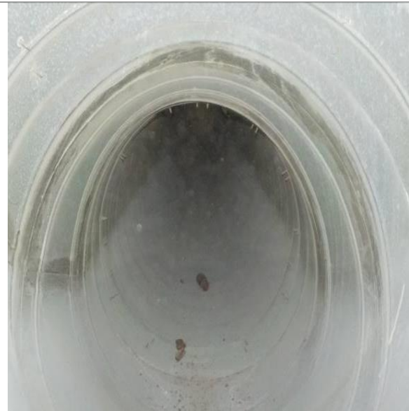
--Before-- Sample of Mechanical Area Ducts
