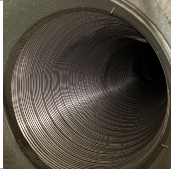
--Before-- Main Duct
