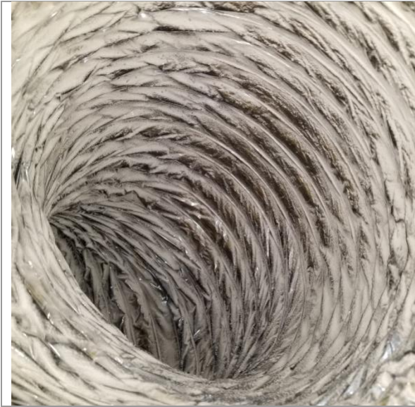
-Before- Dirty flex duct
