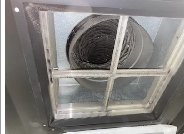
-Before- Dirty flex duct
