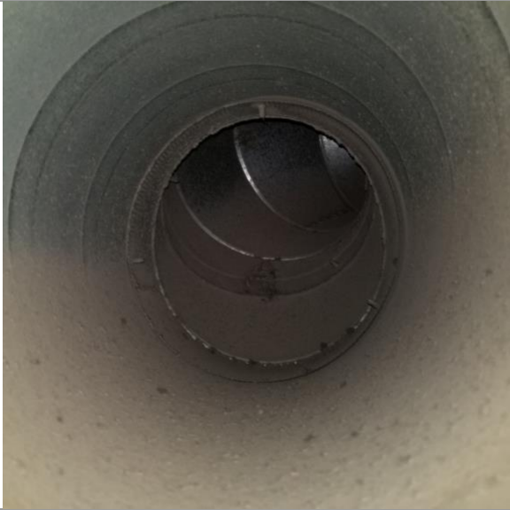
-Before- Dirty main duct
