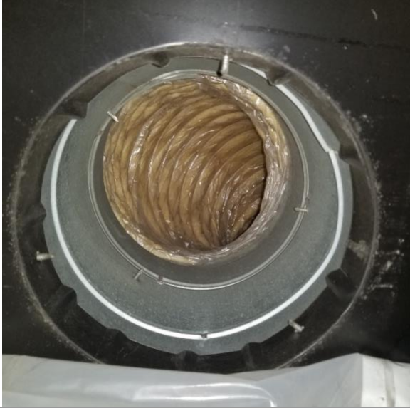
--Before-- Dirty flex duct
