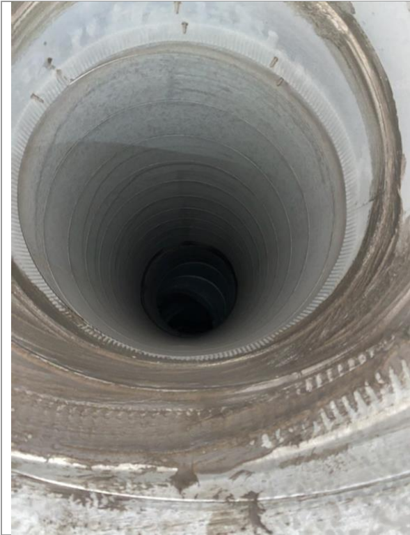
--Before-- Dirty main duct
