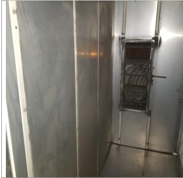
--Before-- Interior of fan compartment with debris
