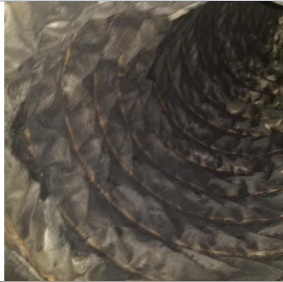
--Before-- Flex duct with heavy debris
