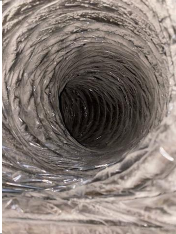
-Before- Dirty flex duct
