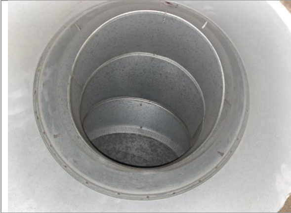
-Before- Dirty duct
