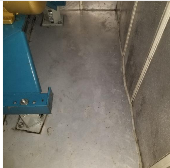
-Before- Fan with debris and organic growth
