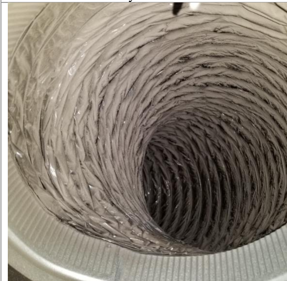
-Before- Dirty flex duct
