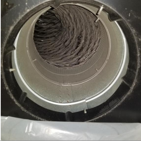
--Before-- Dirty flex duct
