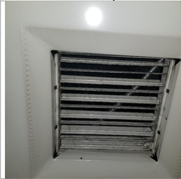
--Before-- Debris on registers
